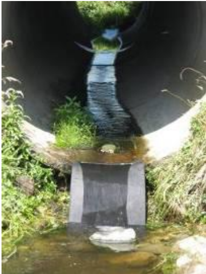
Figure 6: Conveyor belt material bolted on to the outlet end of a culvert in the Aorere catchment to assist fish passage
